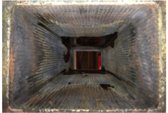
Fig. 8 WAVE mould at end of its life having cast 1795 heats or 50,000 tons
